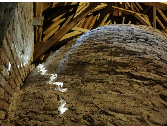
Figure 2. A crack in the vault, Hippolytus Church, Middelstum. Photo credits: OUOU .
