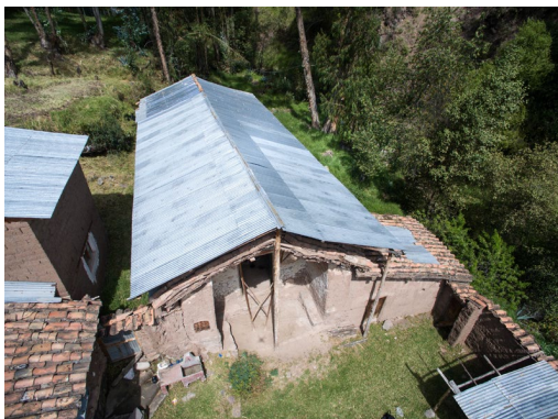
Figure 1. Temporary cover structure to prevent water leaks caused by rain. Source: Own photographs.
