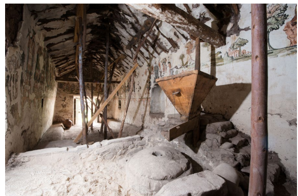
Figure 3. Pair and knuckle in poor maintenance conditions, which causes leaks, humidity that affects and induces discoloration and loss of pictorial layers). Source: Own photographs..
