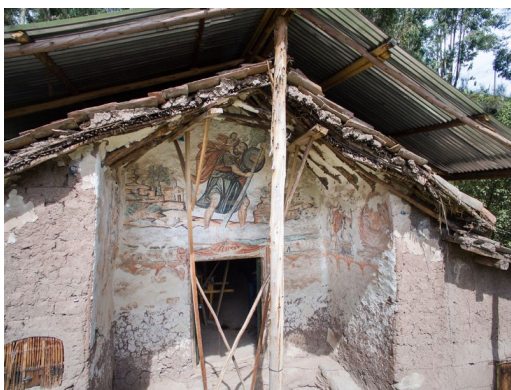
Figure 2. Mural paint on a façade with detachment pathologies produced by direct exposure to environmental factors. Source: Own photographs.
