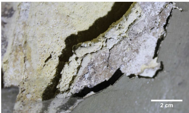
Figure 2. Delamination of the stone extending to the paint layers.
