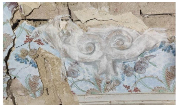
Figure 3. Detachment of a portion of gilded stucco.
